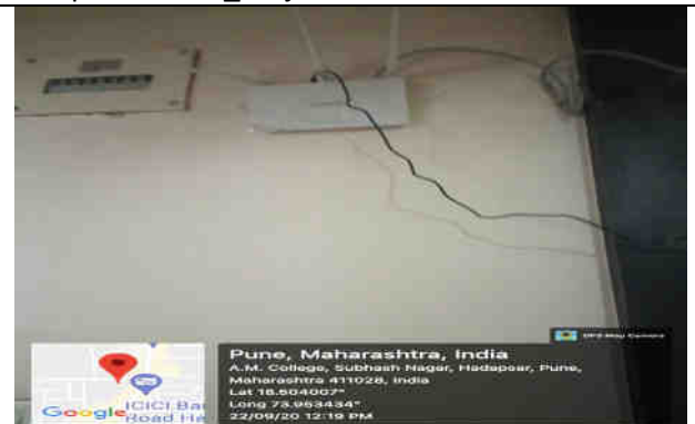
Comp Sci_Wifi Router
