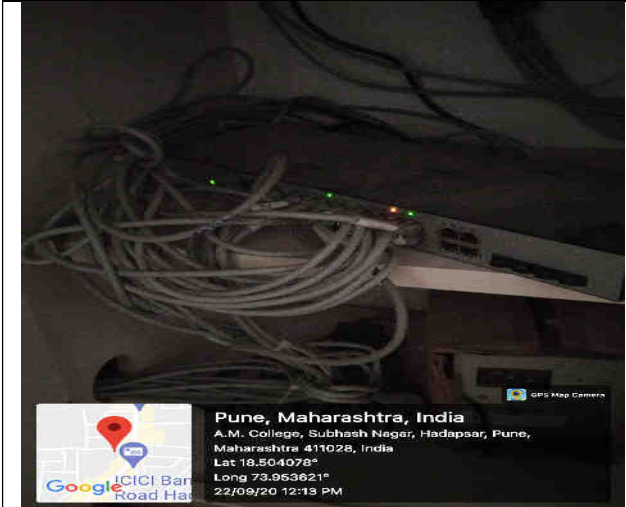
Electronic_24 Port Switch
