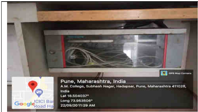
Chemistry_ 24 Port Switch
