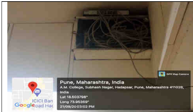
Library_48 Port Switch 2
